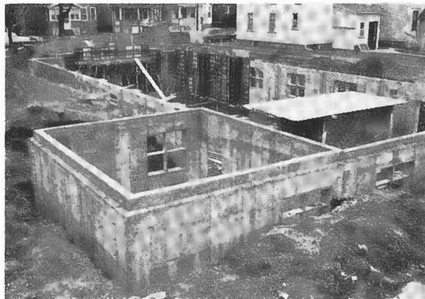
A significant stride is made in building the new structure with completion of the foundation and walls of the church hall early in 1961.
