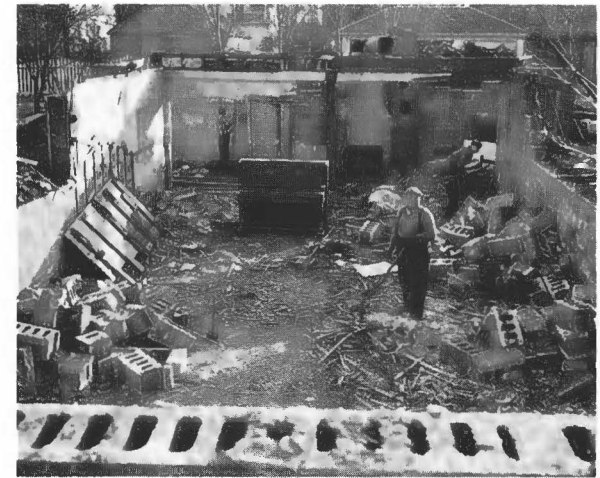
The piano still stands on firm footing as workmen proceed with demolition of the fire ruined structure in November 1960 — first phase of constructing a new church.
