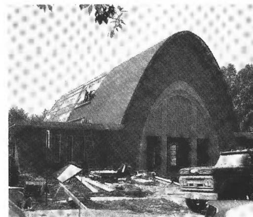
The new church begins to take its final exterior form in the winter of 1961-2.
