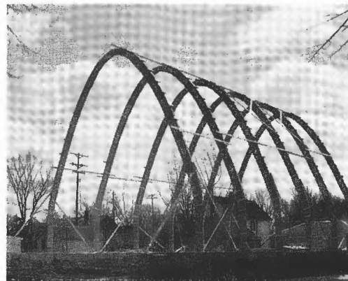
Work proceeds on schedule and the parabolic arches of the modern Byzantine design are erected in the Spring of 1961.
